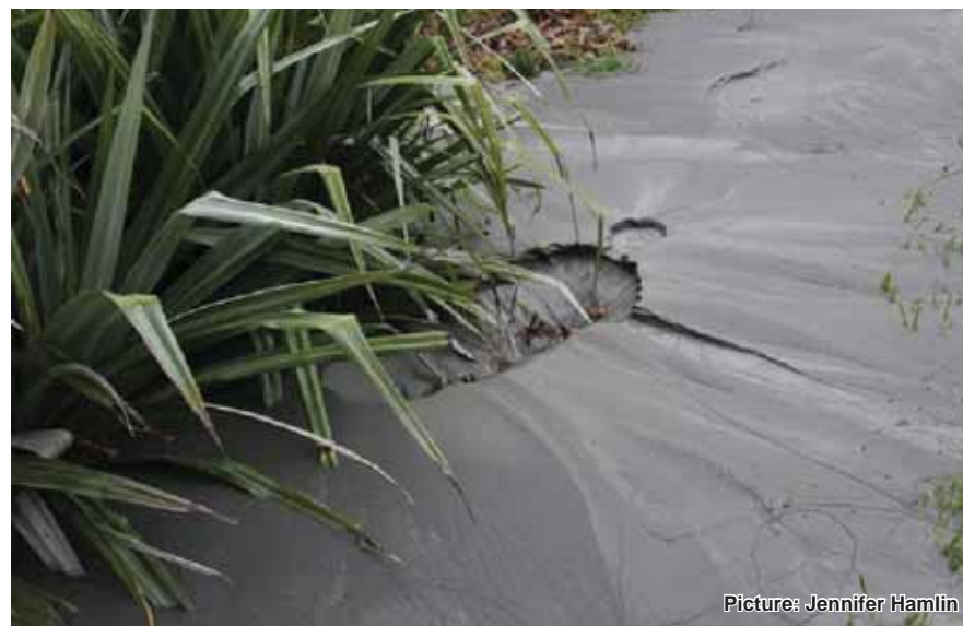
Liquifaction of the footpath.
